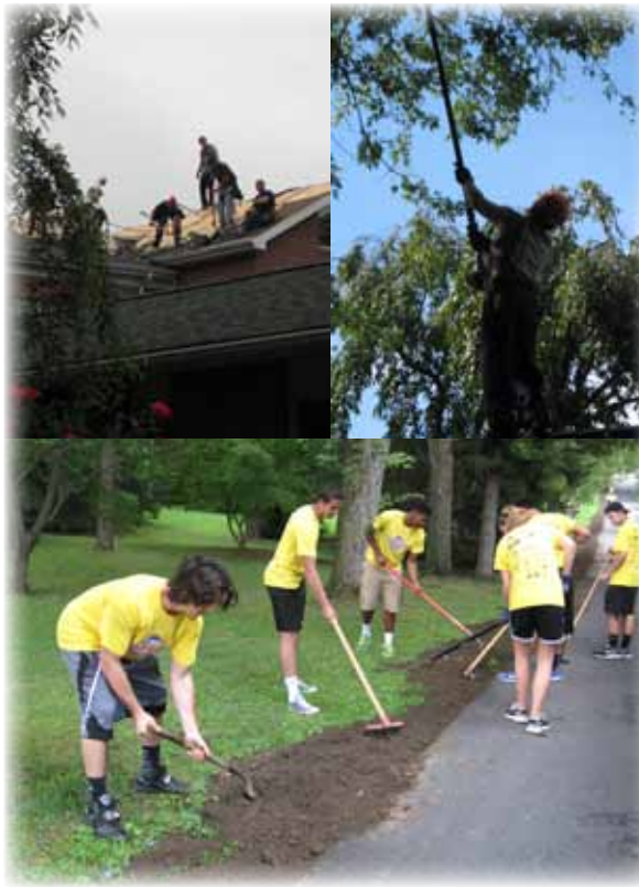
Clockwise: Roofers, Bob on the roof with his chainsaw, and the students from St Vincent.
